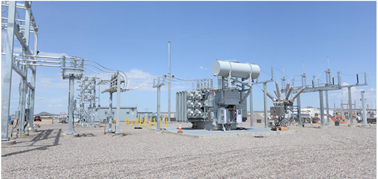
Figure 3: Example of Eskom substation
