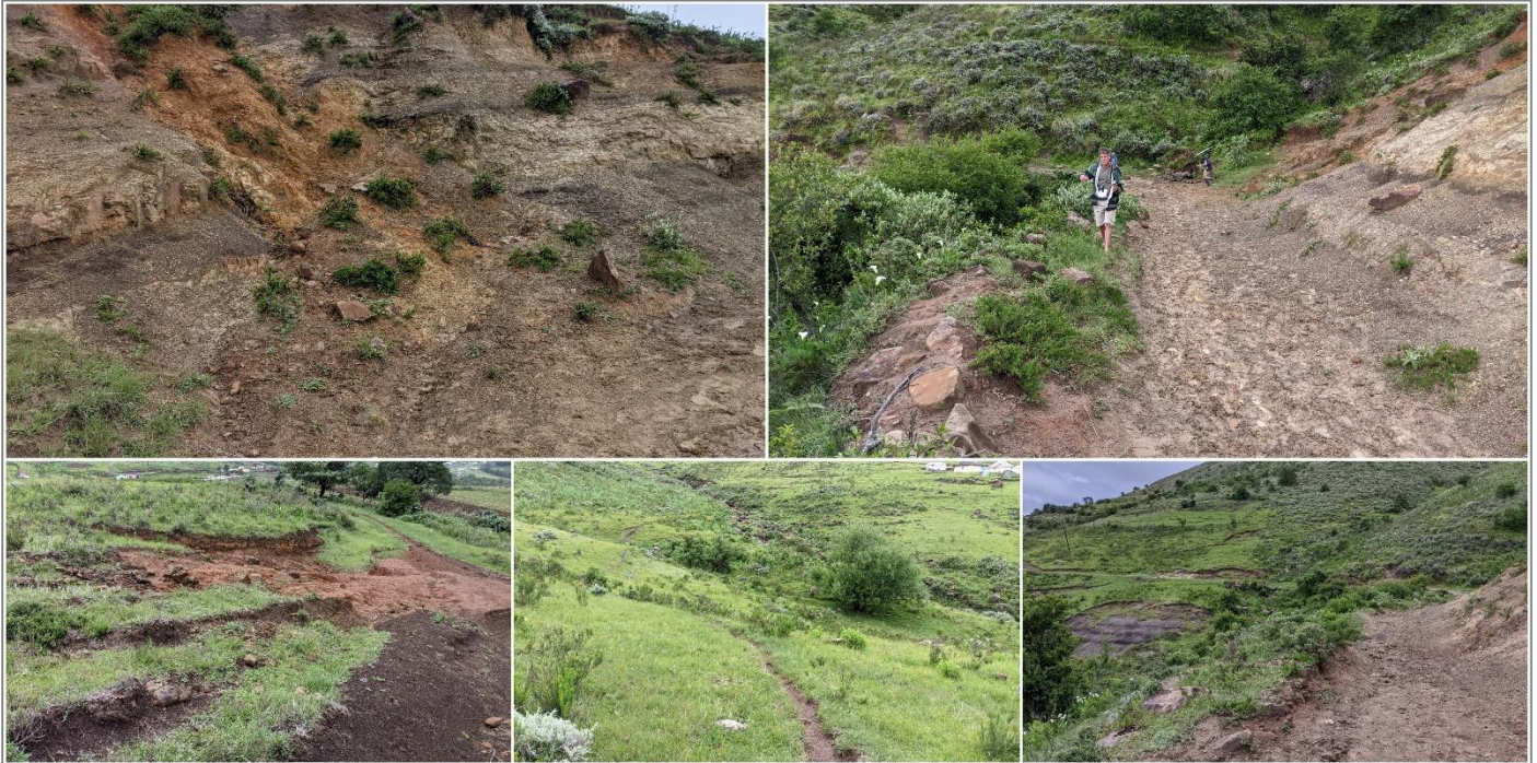
Figure 13 Erosion present along the proposed road extension
