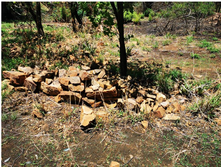
Figure 22: Collapsed walling at UP-BAV-2528-02
