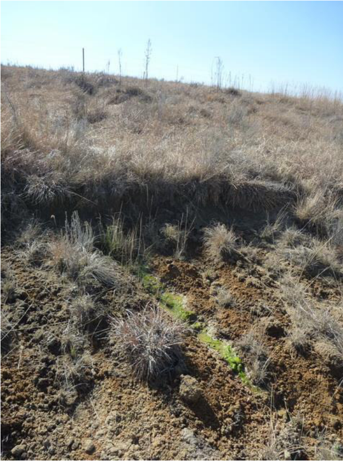
Figure 23 Road cutting with exposed flow (outside of a wetland area) at the end of July 2013
