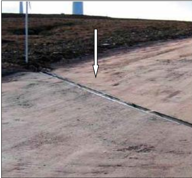
Figure 2-3: Cross drains under the Internal Roads
