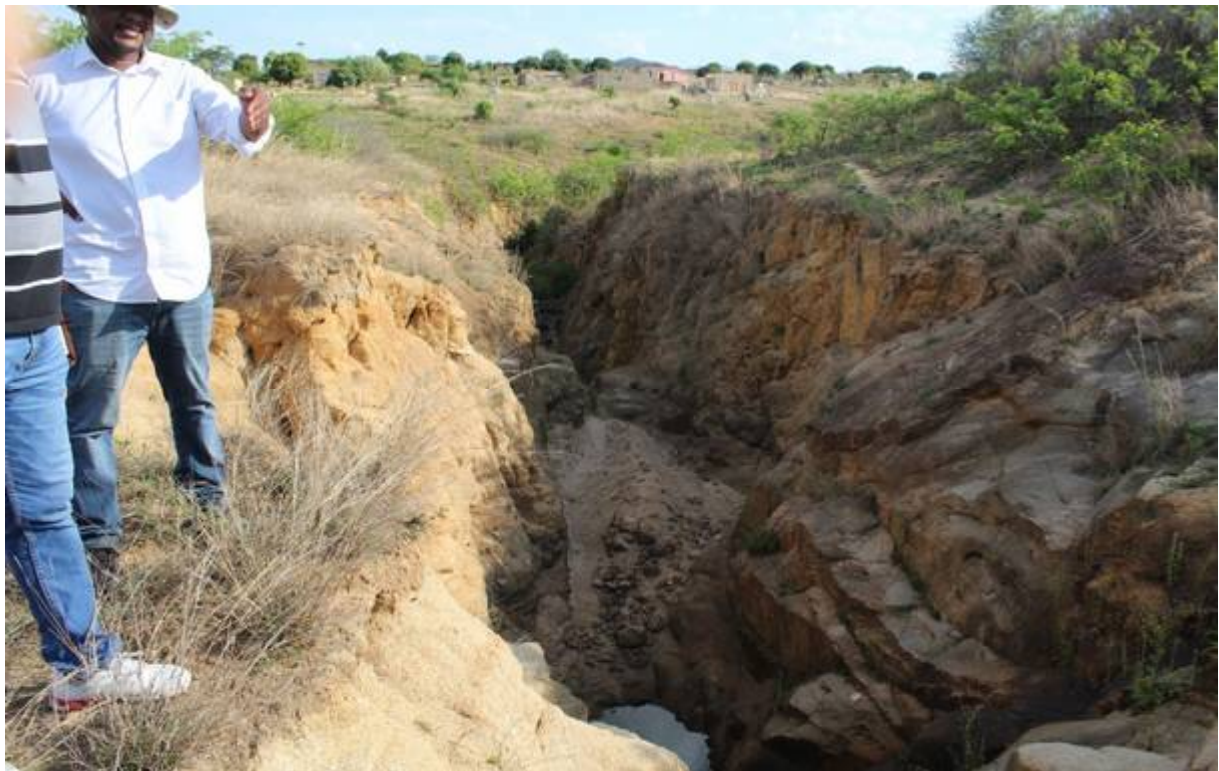
Figure 5: Delegates inspecting the large donga below the spillway of Casteel Dam.
