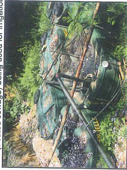
The current sewage treatment facility
