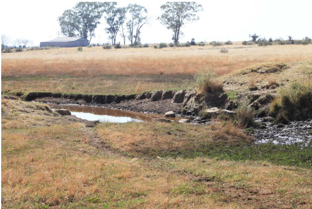
Broken groundwall of small in-channel dam at the northern boundary of the site. Photo: R.F. Terblanche
