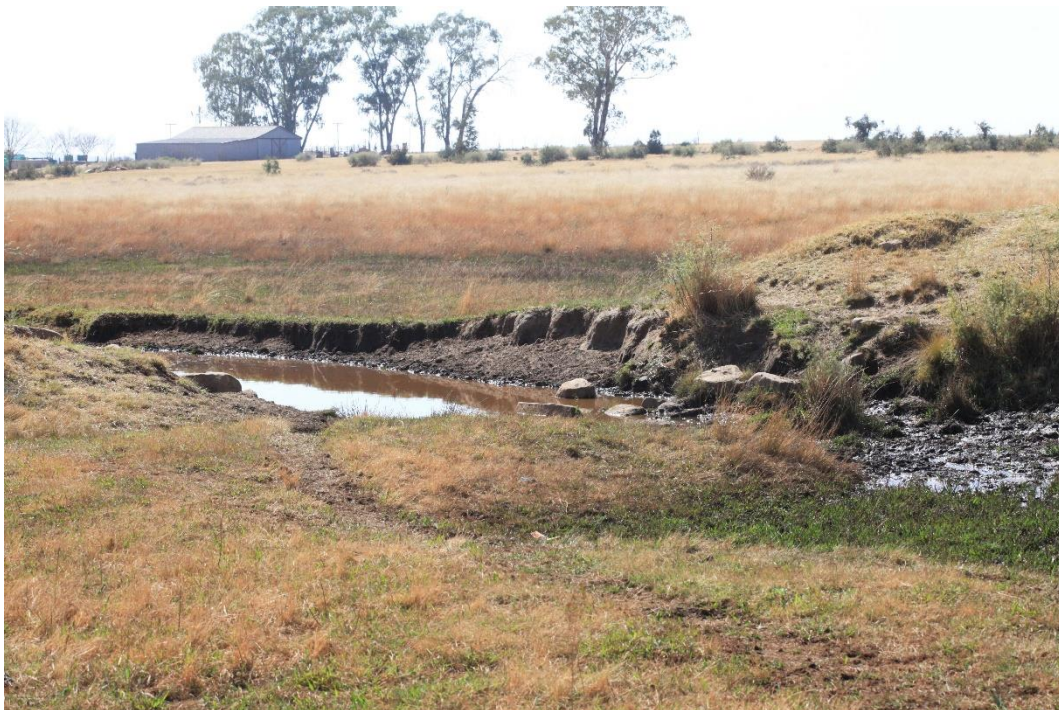
Photo 6 Broken groundwall of small in-channel dam at the site. Photo: R.F. Terblanche
