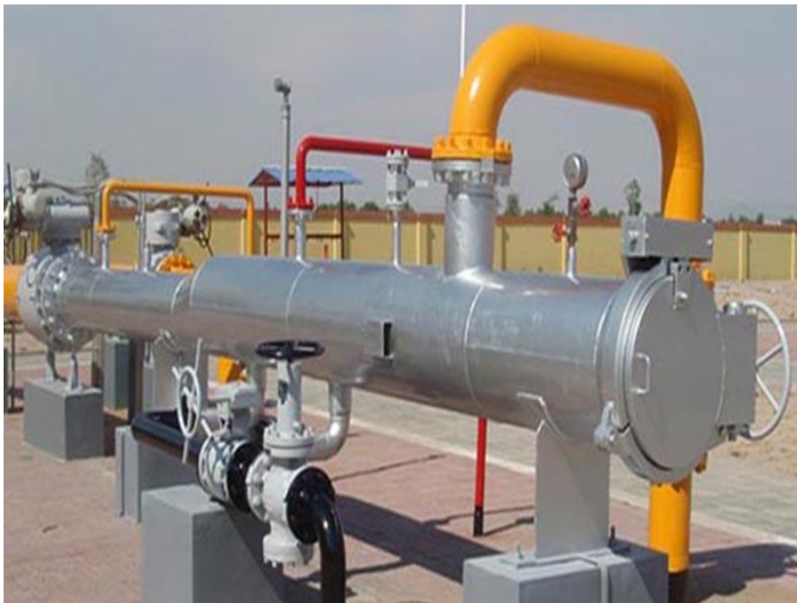
Figure 2-2 – Pig launcher/receiver for a natural gas pipeline
