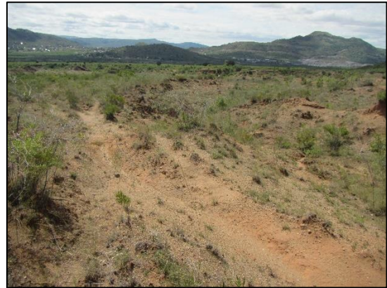
Figure 13: Sparsely vegetated eroded gullies.
