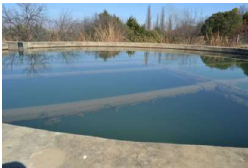
Figure 8: Launder pipes installed within clarifier
