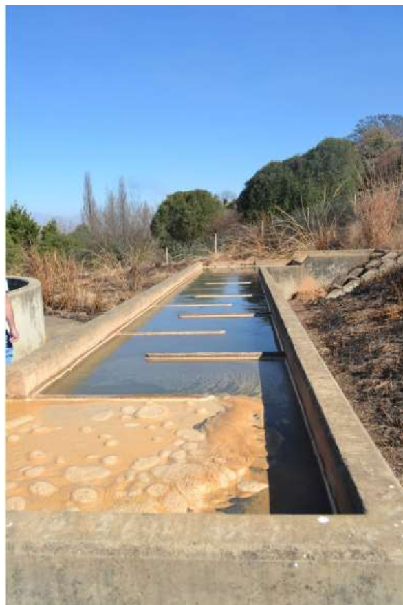
Figure 6: Lower section of flocculation channel
