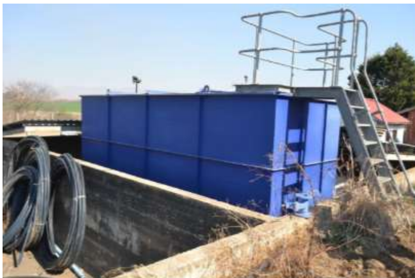
Figure 14: Existing package treatment plant
