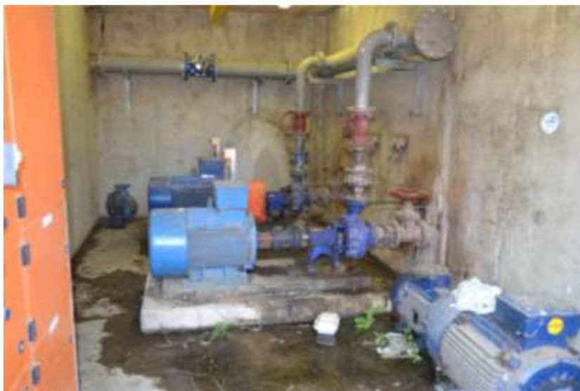
Figure 13: Clearwater pump station pumps and pipework
