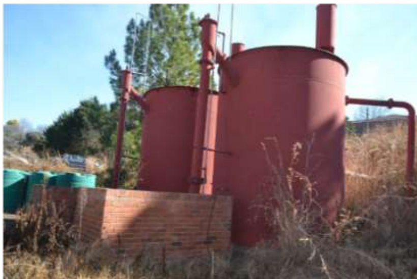
Figure 9: Auto-backwash gravity filters
