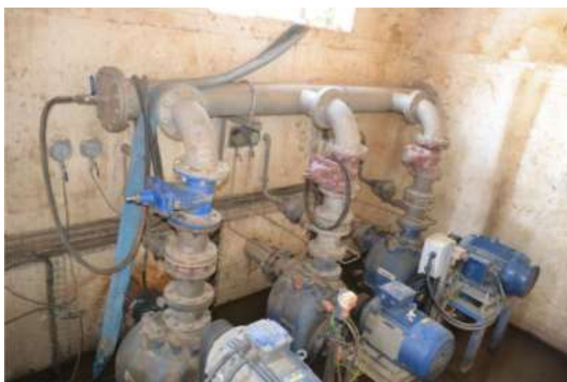
Figure 2: Raw water pump station pumps and pipework
