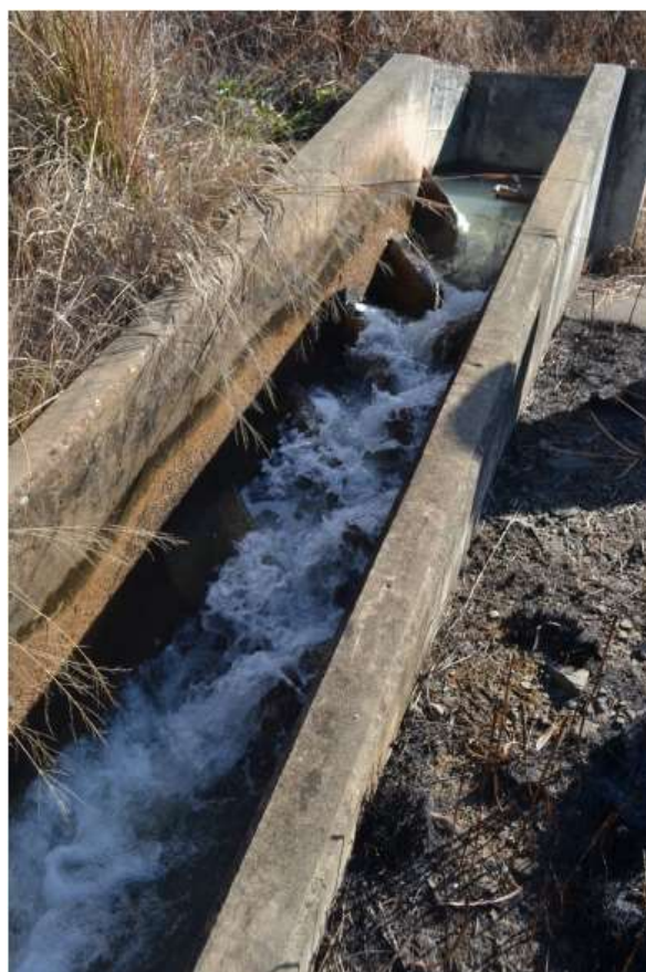
Figure 5: Upper (sloped) section of flocculation channel
