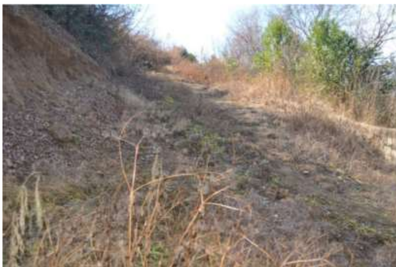
Figure 16: Access road to raw water pump station is in a state of disrepair
