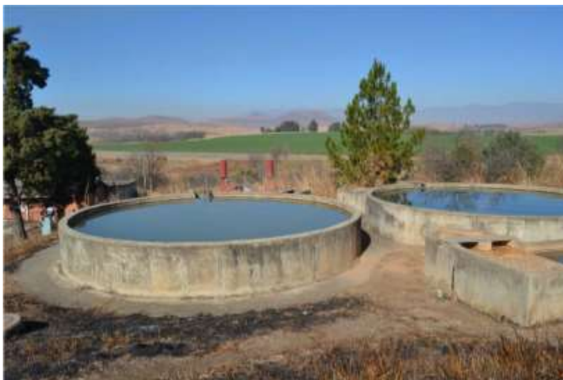
Figure 7: Circular sedimentation tanks
