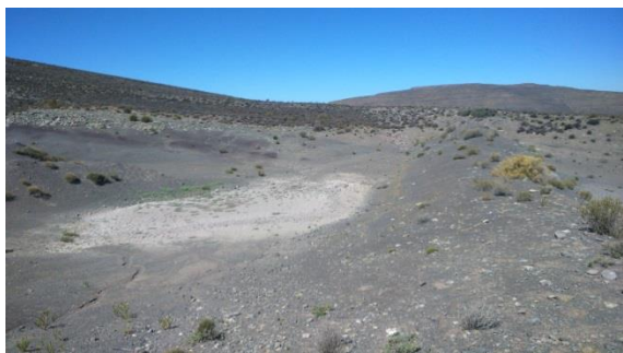
Plate 7: Broken Earth-wall dam
