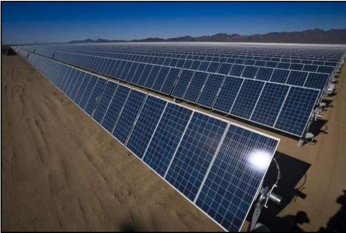
Photograph 1.1: Typical PV SEF facility
