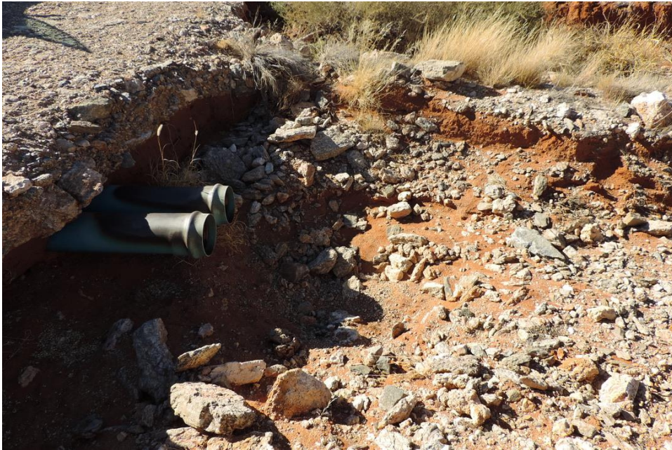
Figure 9 Old water flow infrastructure at a preferential flow path crossing along an existing farm road
