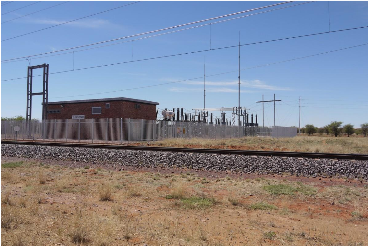
Plate 1, View of Emil Switching Station from VP1.
