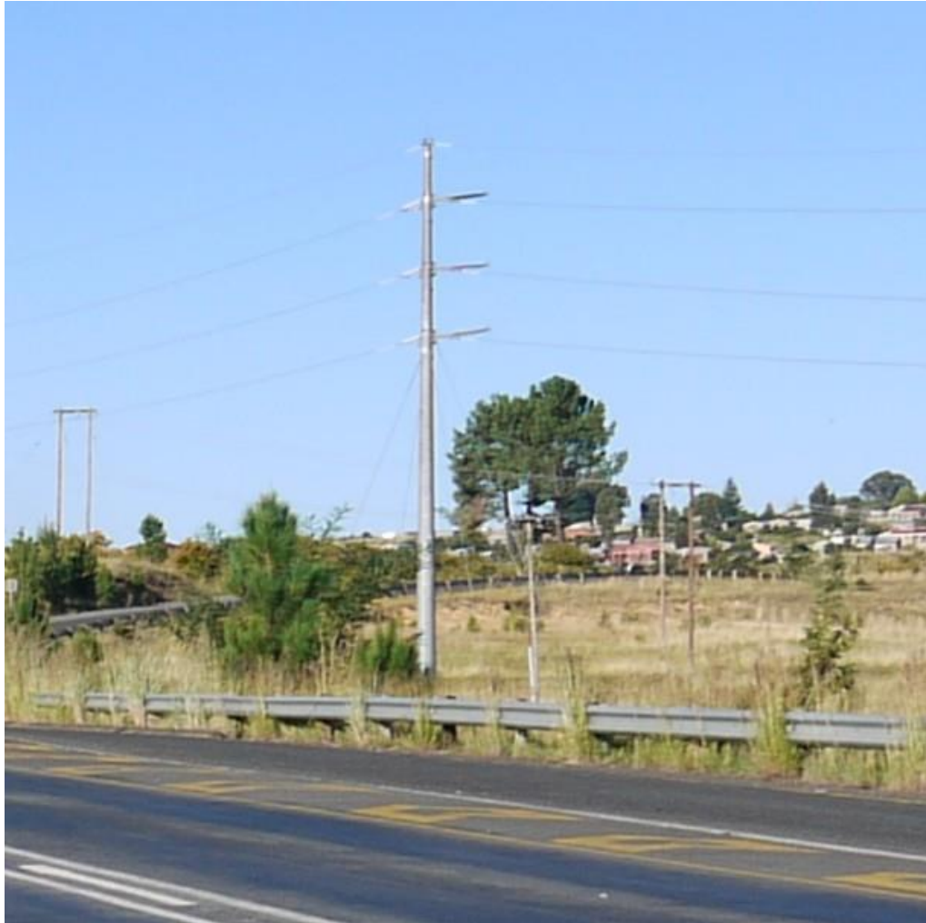
Plate 3, Typical 23-28m high 132kV self-sustaining steel monopole tower.
