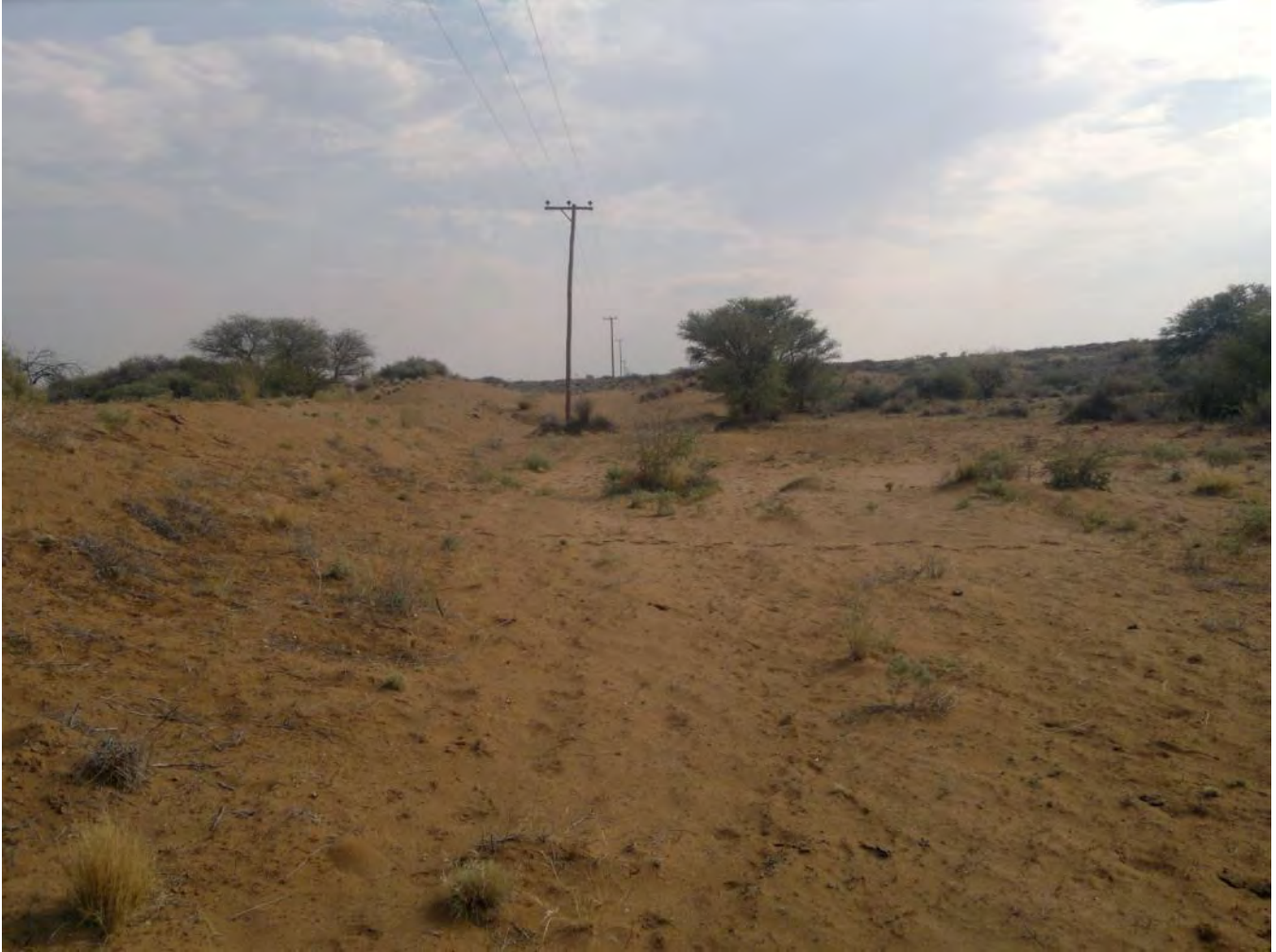
Figure 16 – Berm / impounding wall (left) constructed across the width of the watercourse at Crossing Alt1_13, with area behind in which water is trapped
