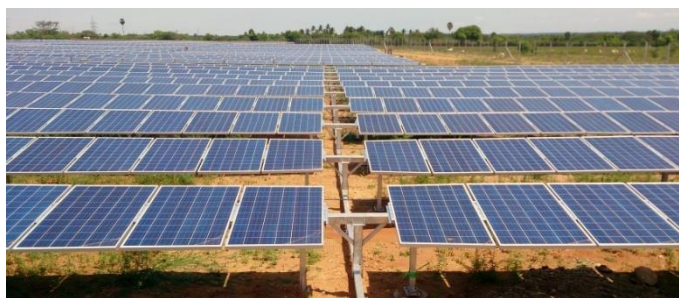
Figure 1: Single axis solar PV module tables raised 500mm above ground level
