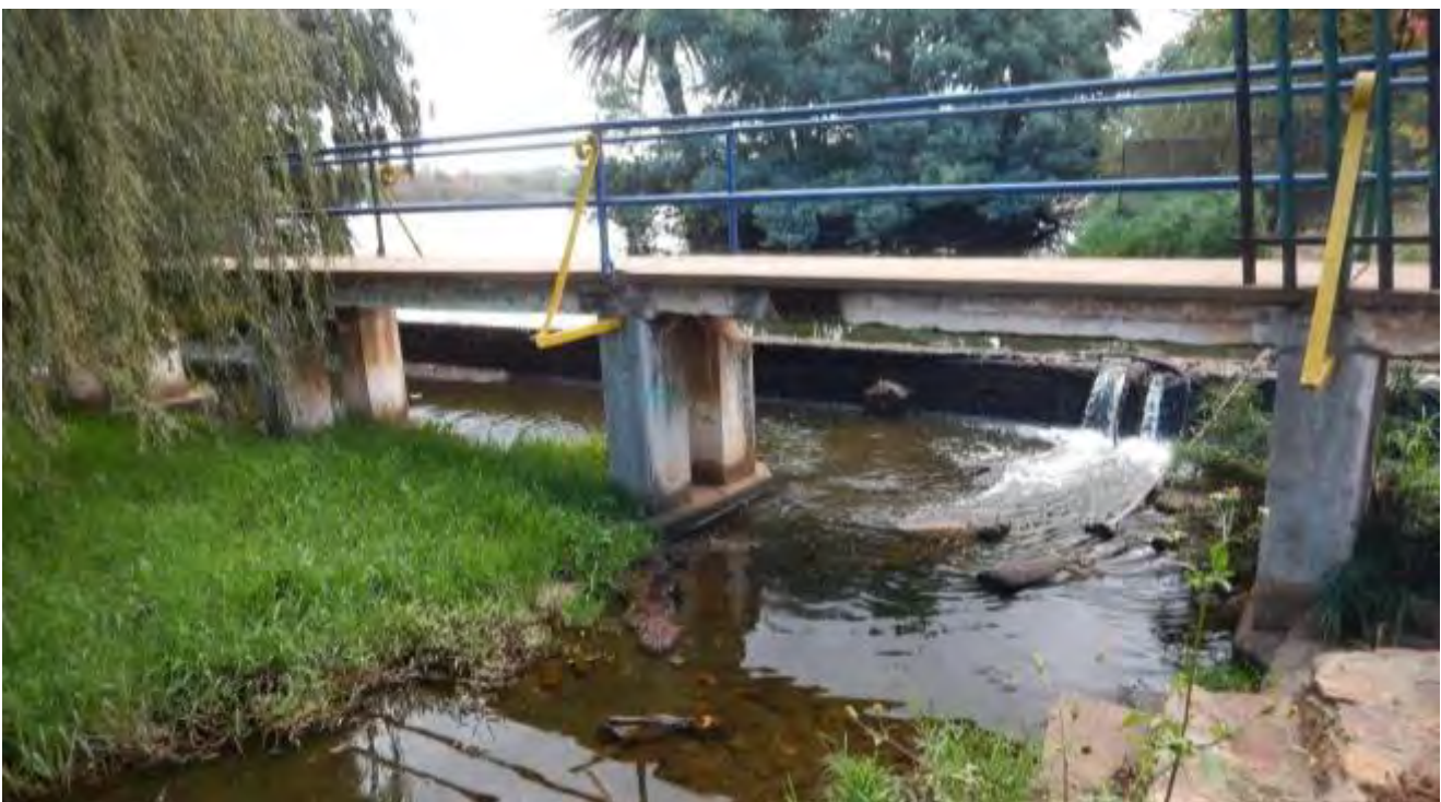
FIGURE 2-9: OVERFLOW OF FLORIDA LAKE
