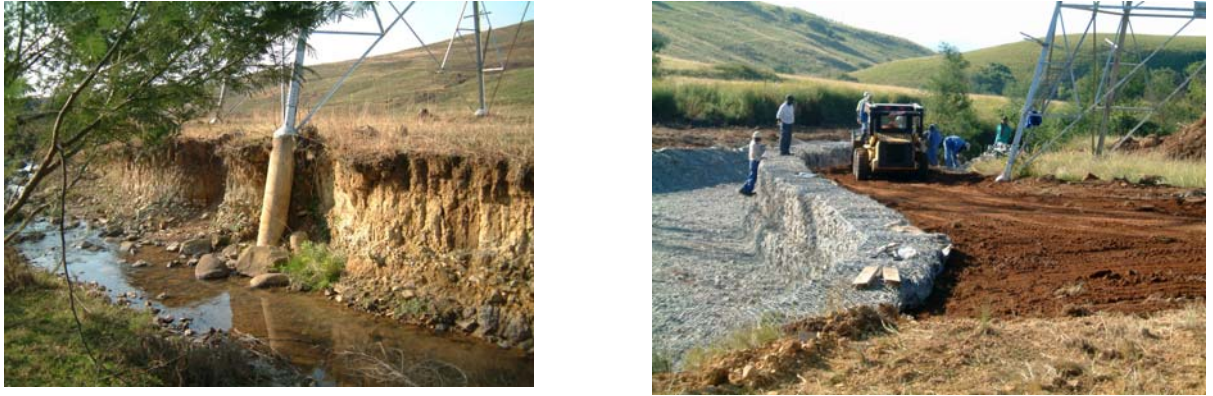
Figure 1: The photo on the left shows the foundation of a tower exposed by erosion. The photo on the right shows the extensive and costly remediation by using gabions and reno mattresses. Also note the use of good topsoil that will permit the re-establishment of vegetation around the tower (photos JorgeCorreia).
