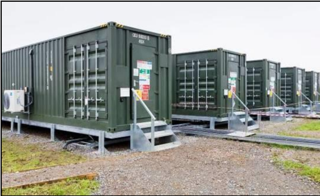
Photograph 1.2: Example of BESS located in storage containers
