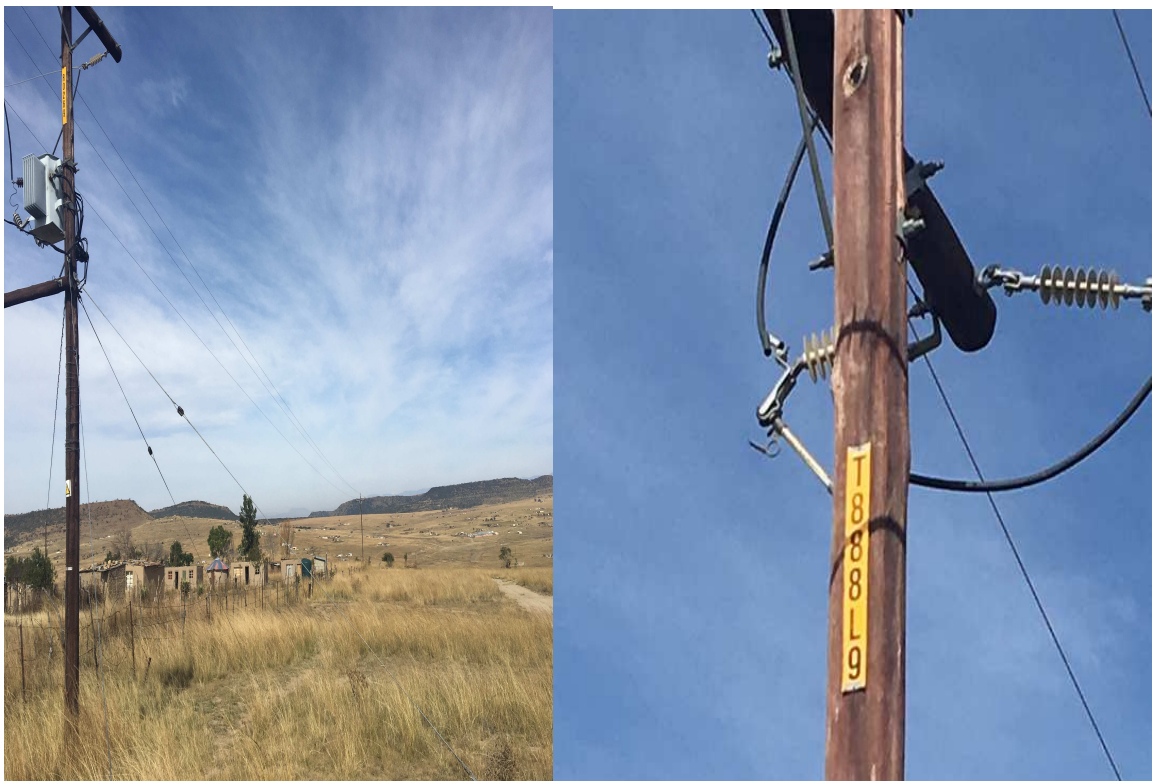
Figure 4: Existing Eskom 11kV MV Infrastructure
