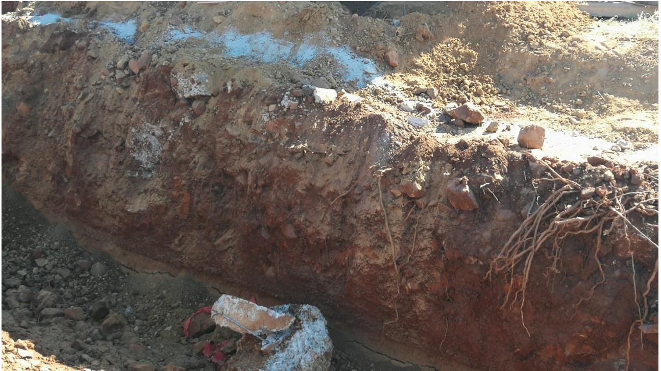
Figure 17: Soil characteristics of the proposed PSTs area in an excavated trench. Note the rocky red soil with no grey matrix or mottling.
