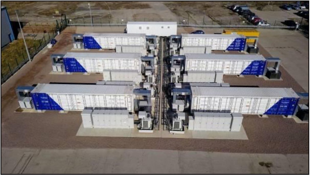
Photograph 1.2: Example of BESS located in storage containers
