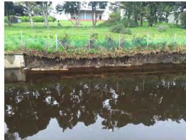
Photo P Broken section of the canalised eastern channel of the Liesbeek, showing collapsed canal liners on the right hand river bank
