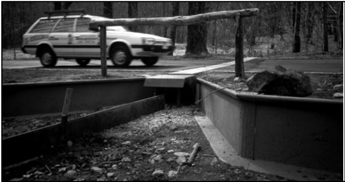
Figure 22: An example of an underpass with a grid roof, designed for toads and other small faunal species. The entrance/exit points are fringed with steep-sided walls to direct faunal movements.
