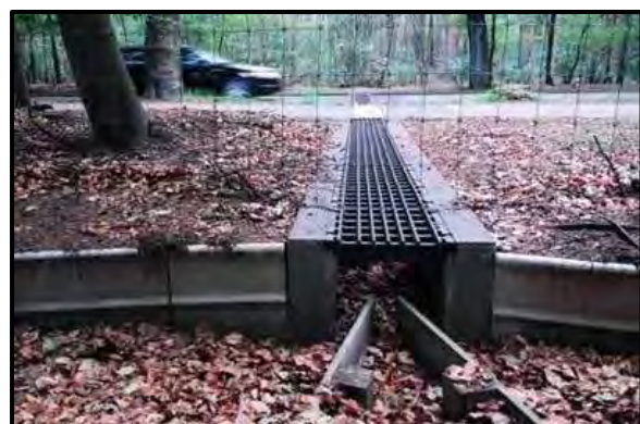
Figure 26: Underpass with a grid roof, designed for toads and other small faunal species.
