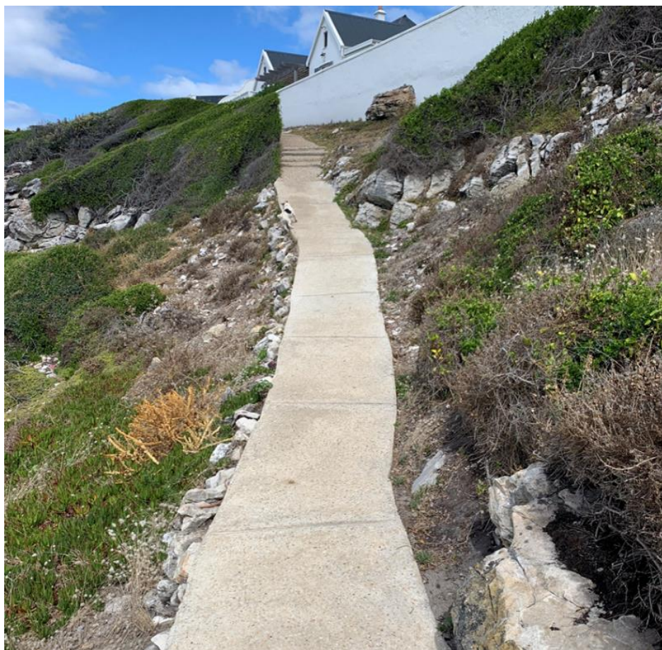
Figure 1 A section of the current Hermanus Cliff Path near the proposed site (Anchor 2021).
