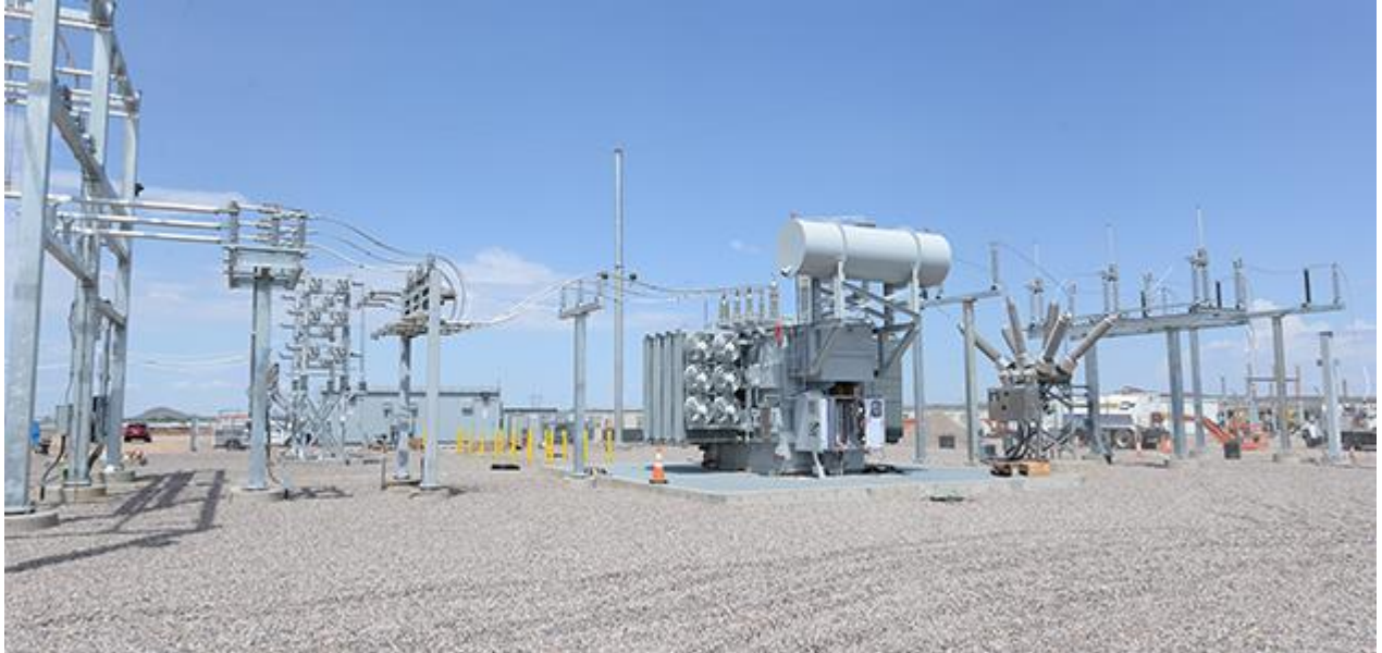
Figure 1-4: Example of substation
