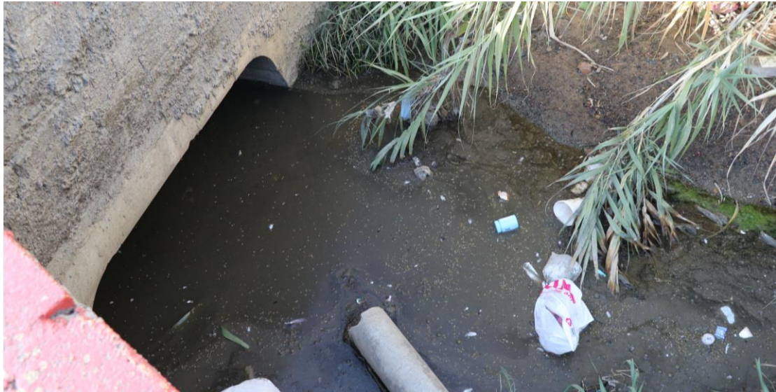
Figure 9: Where the storm water channel enters the site, it emerges from an underground section. Water quality is quite clearly very poor.
