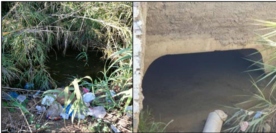
Figure 9: Photographic evidence during the site visit of the storm water drain on site.
