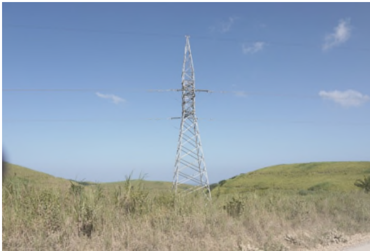
Plate 3, Eskom 132kV Lattice Tower 25-28m high. 132kV structures will be slightly higher than existing and will follow the existing power line servitude.
