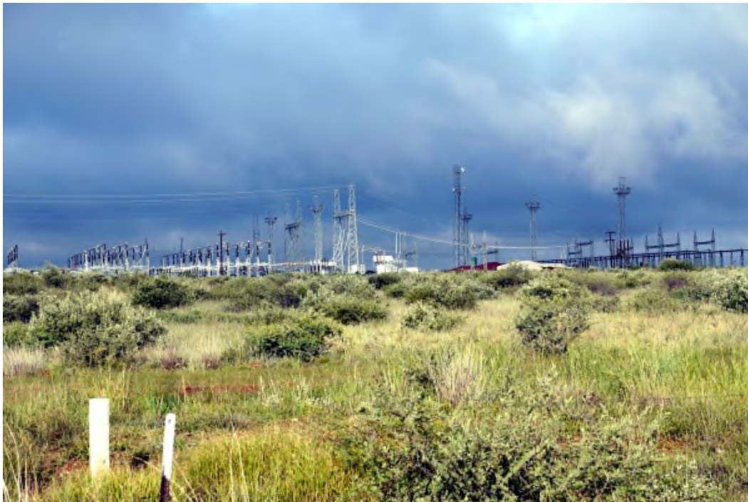
Plate 1, Existing Mookodi 400/132kV Substation.
