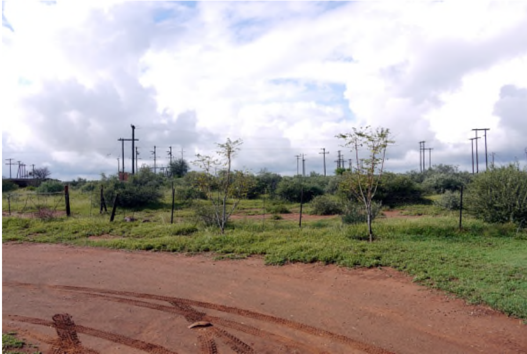
Plate 2, Existing Eskom MV overhead powerline on the northern boundary of the site. A number of alternatives are under consideration for the necessary grid connection which are subject to Eskom's plans for the construction of a new substation (Bophirima) in the area indicated as well as a new 132kV overhead power line link to the existing Mookodi Substation. The proposed internal power line will be viewed in the context of this infrastructure.
