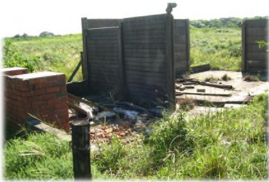
Photo 9. Old dilapidated building probably linked to the old airfield.
