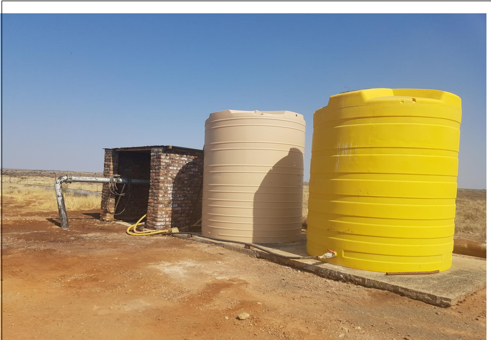
Figure 15: Extraction Pump for Pivot 8 from pipeline (29°35'8.33"S; 24° 4'54.54"E)
