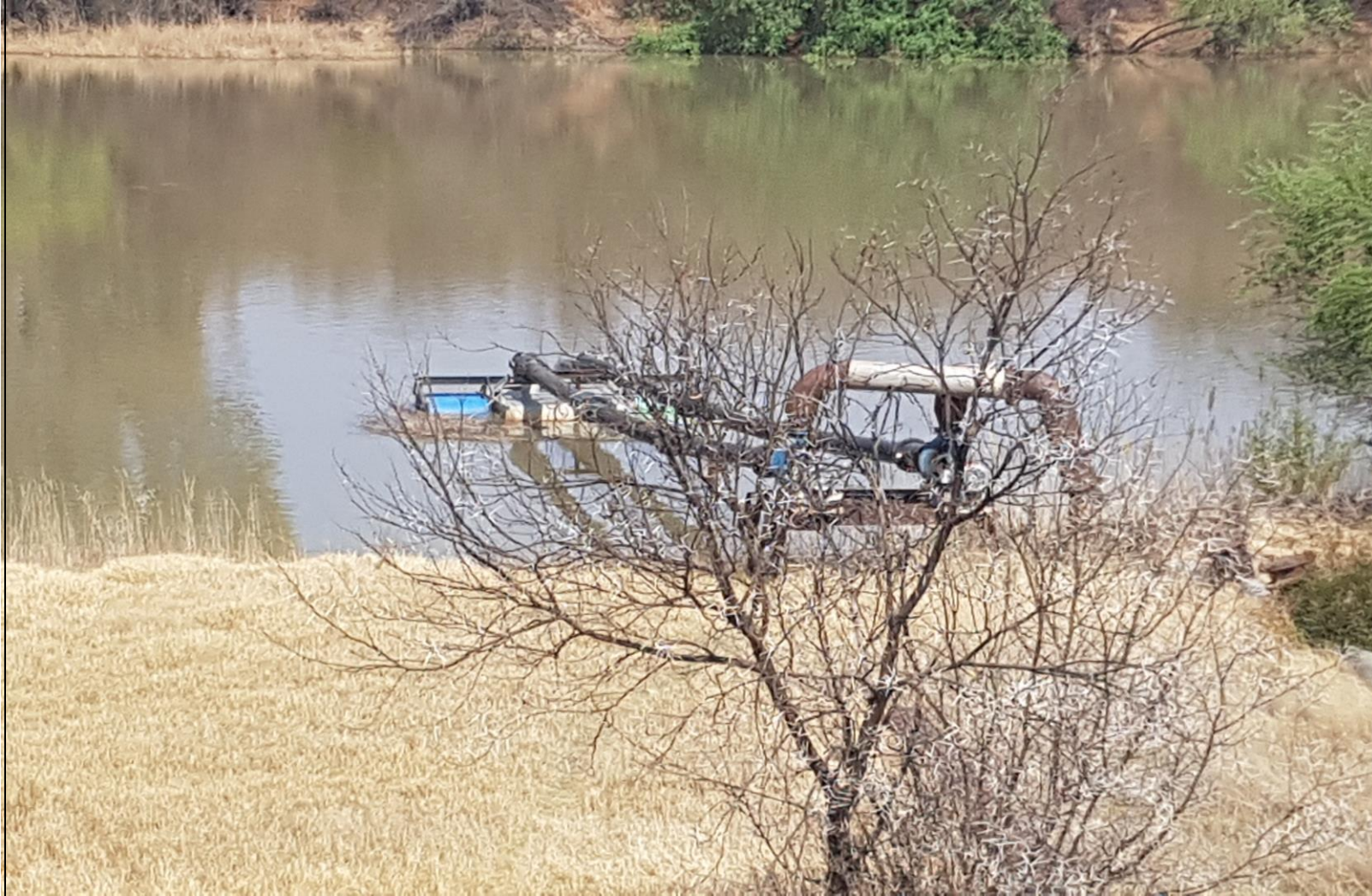
Figure 21: South-easterly Extraction pump from Orange River (29°35'23.55"S; 24° 4'39.05"E)
