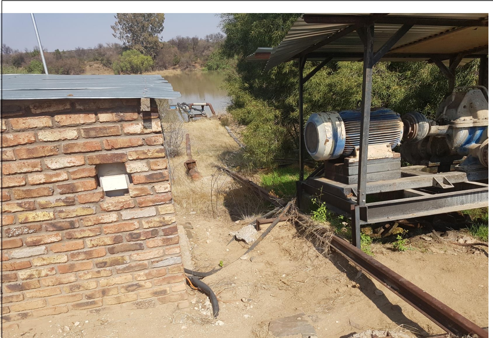
Figure 20: South-easterly Extraction pump from Orange River (29°35'23.55"S; 24° 4'39.05"E)
