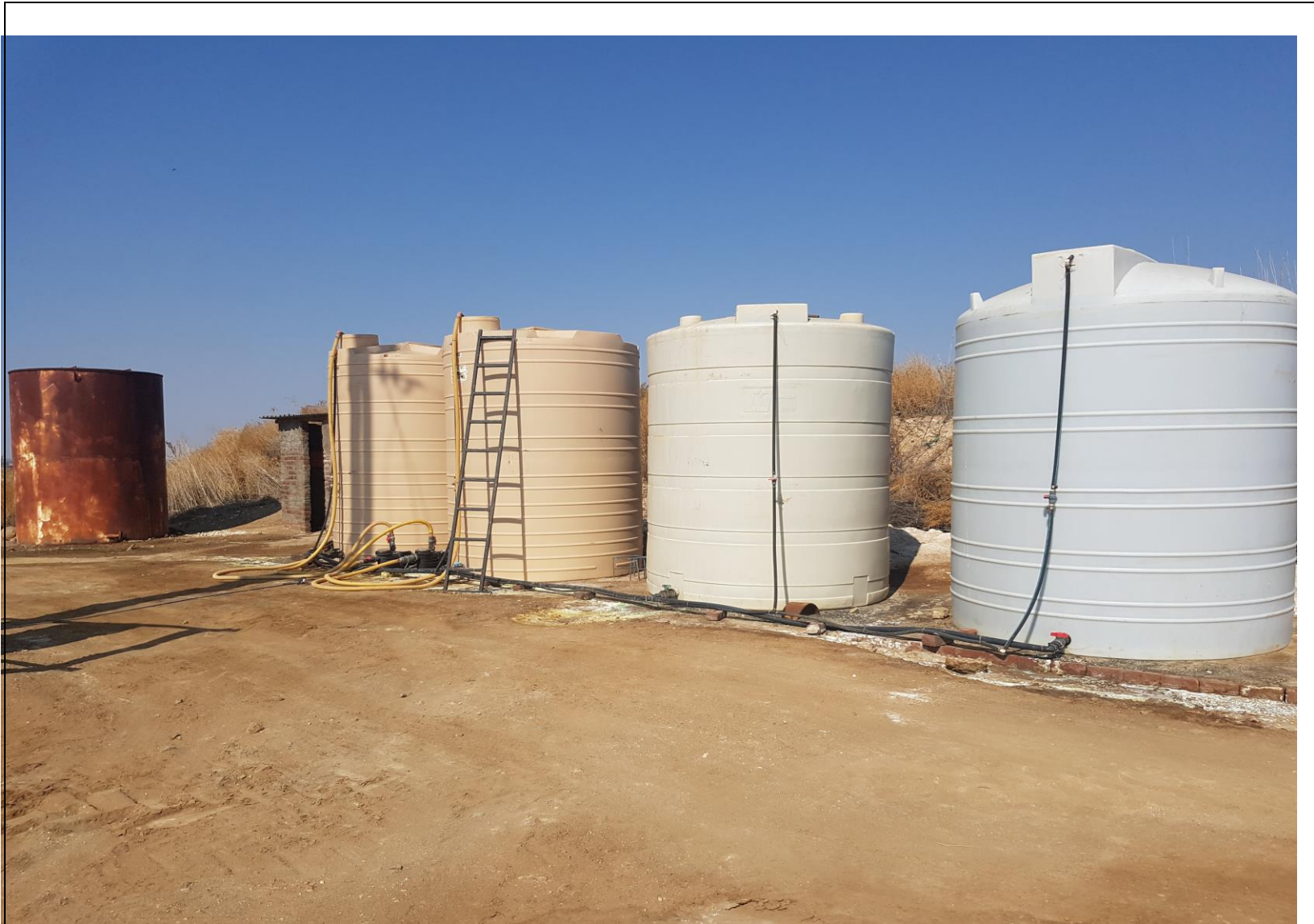
Figure 7: Pivot 11 and 12 Extraction pump from Dam (29°34'44.93"S; 24° 5'18.95"E)
