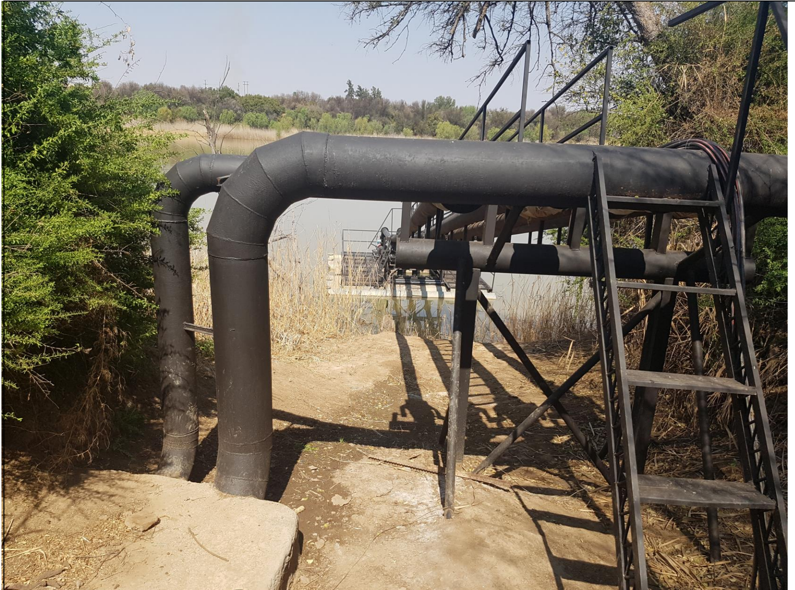
Figure 22: South-Westerly Extraction pump from Orange River (29°35'43.99"S; 24° 6'15.06"E)
