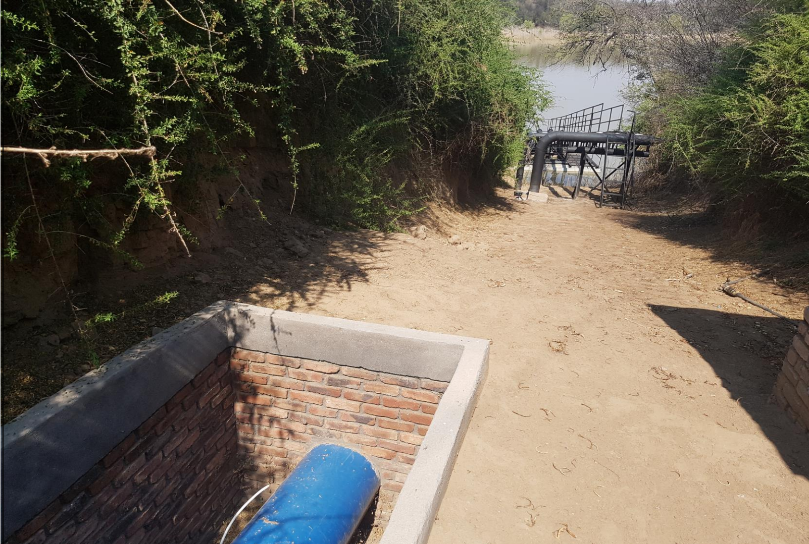
Figure 23: South-Westerly Extraction pump from Orange River (29°35'43.99"S; 24° 6'15.06"E)
