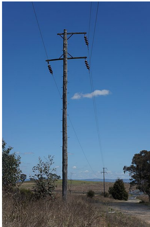
Figure 2: Image of a typical 66kV Powerline Tower 3
