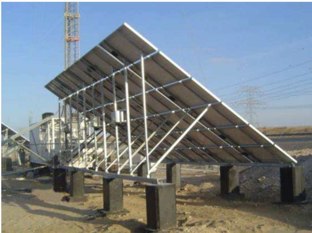
Plate 4, PV array viewed from behind and the side. The dark face of the PV units are not obvious and subject to the colour of the undersides of the units, the supporting structures are likely to become more apparent. This might appear as a long industrial structure from close quarters. From a distance however, the shadow cast by the structure will be read and will probably appear similar in nature to the front view of the array.
