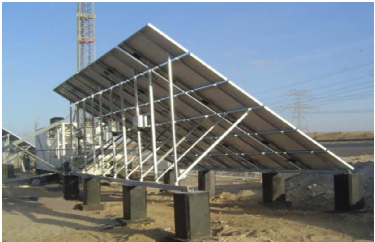
Plate 19, PV array viewed from behind and the side. The dark face of the PV units are not obvious and subject to the colour of the undersides of the units, the supporting structures are likely to become more apparent. This might appear as a long industrial structure from close quarters. From a distance however, the shadow cast by the structure will be read and will probably appear similar in nature to the front view of the array.
