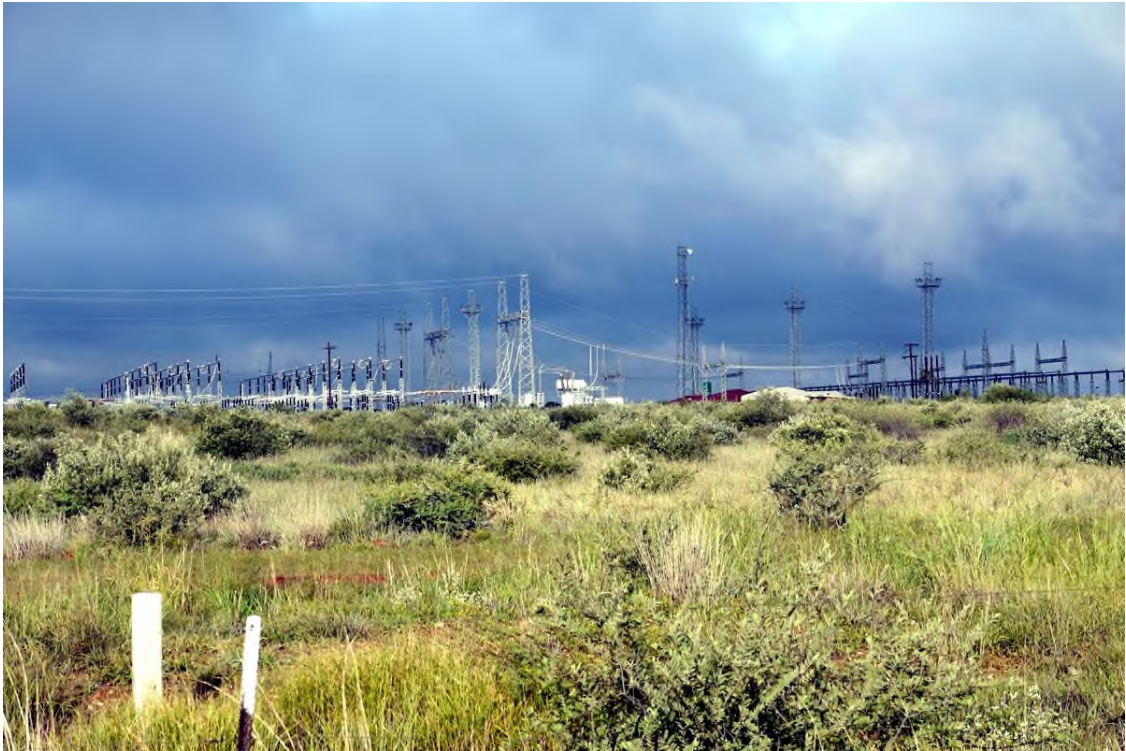
Plate 1, Existing Mookodi 400/132kV Substation.
