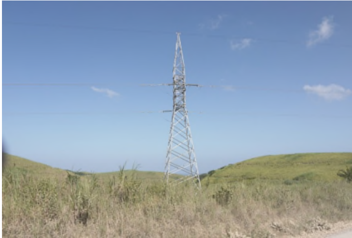
Plate 3, Eskom 132kV Lattice Tower 25-28m high. 132kV structures will be slightly higher than existing and will follow the existing power line servitude.
