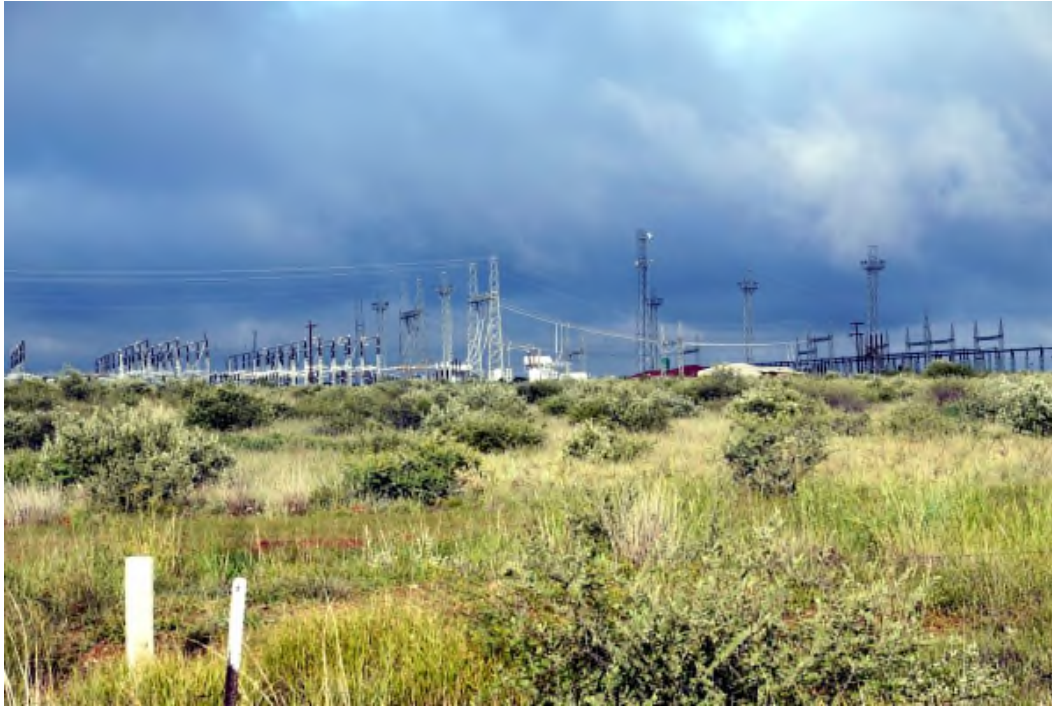
Plate 1, Existing Mookodi 400/132kV Substation.
