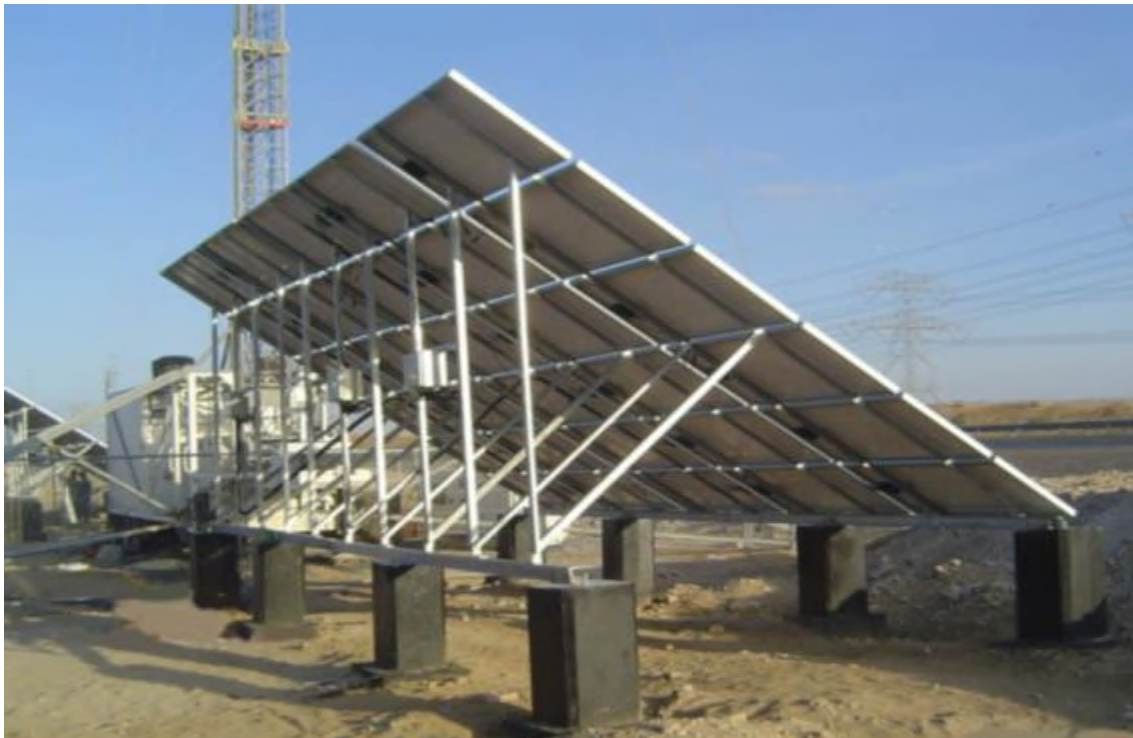
Plate 19, PV array viewed from behind and the side. The dark face of the PV units are not obvious and subject to the colour of the undersides of the units, the supporting structures are likely to become more apparent. This might appear as a long industrial structure from close quarters. From a distance however, the shadow cast by the structure will be read and will probably appear similar in nature to the front view of the array.
