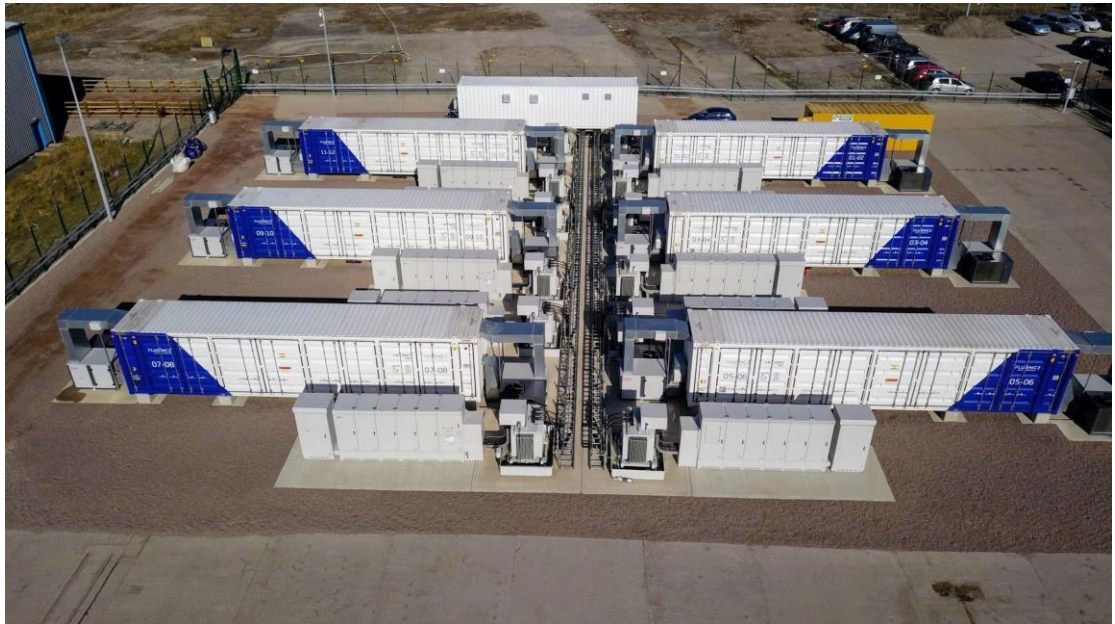
Figure 4: Aerial view of a BESS facility (Photo: Power Engineering International).
