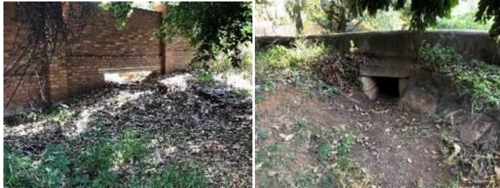
Figure 16 & 17: The opening in the boundary wall to Erf 348 and the culvert under the unnamed road.
