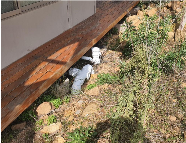
Individual units connected to sewer mains
