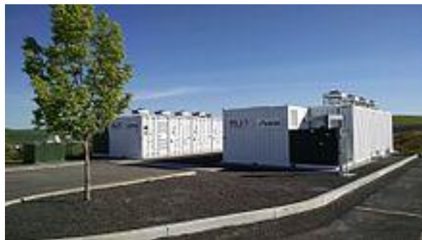
FIGURE 2.3.2.1 – Images of Some Redox Flow BESS Systems – containerized systems or buildings with tanks of electrolyte and battery systems
