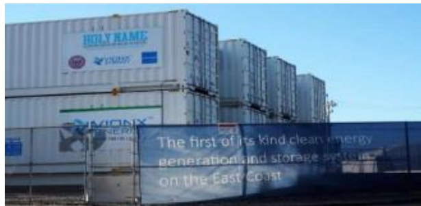
Source – Bushveld Minerals and Energy – Energy Storage and Vanadium Redox Flow batteries 101 – 13 November 2018.
