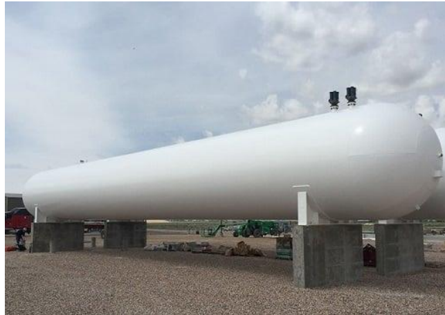
Figure 4-11: Bullet storage tank (ammonia storage)
