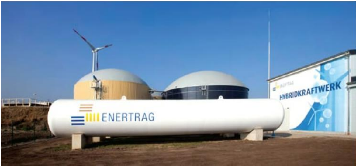
Figure 4-14: Compressed Hydrogen Storage – horizontal tank
