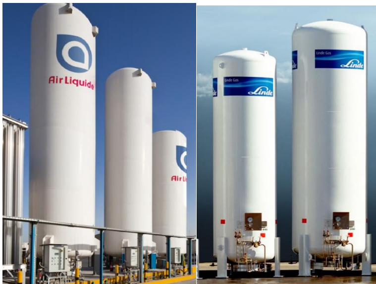
Figure 4-15: Cryogenic storage tanks – vertical tanks.
