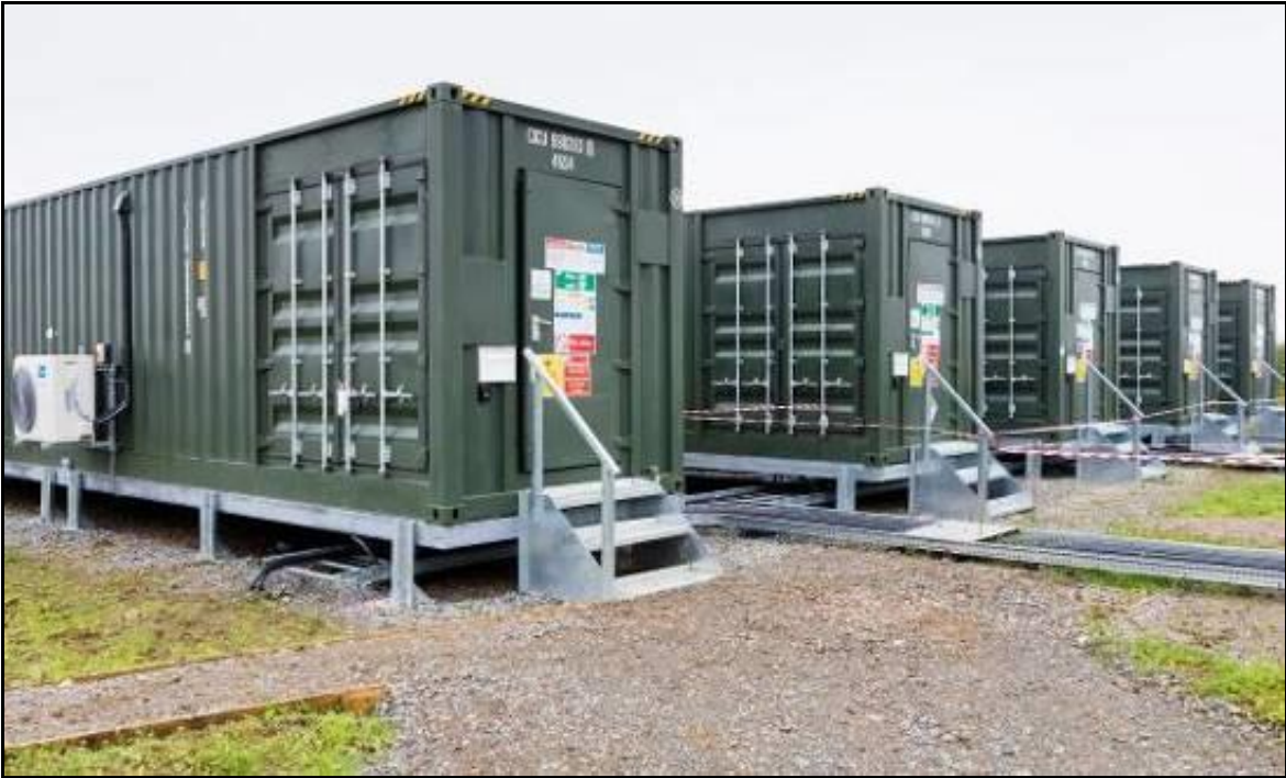
Photograph 1.2: Example of BESS located in storage containers
