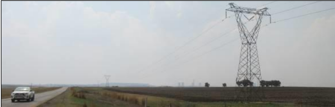
Photograph 3.6: Transmission line along the R546 on Vantondershoek 317/1 (Steyn)
