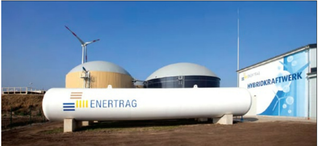
Figure 3-7: Compressed Hydrogen Storage – horizontal tank
