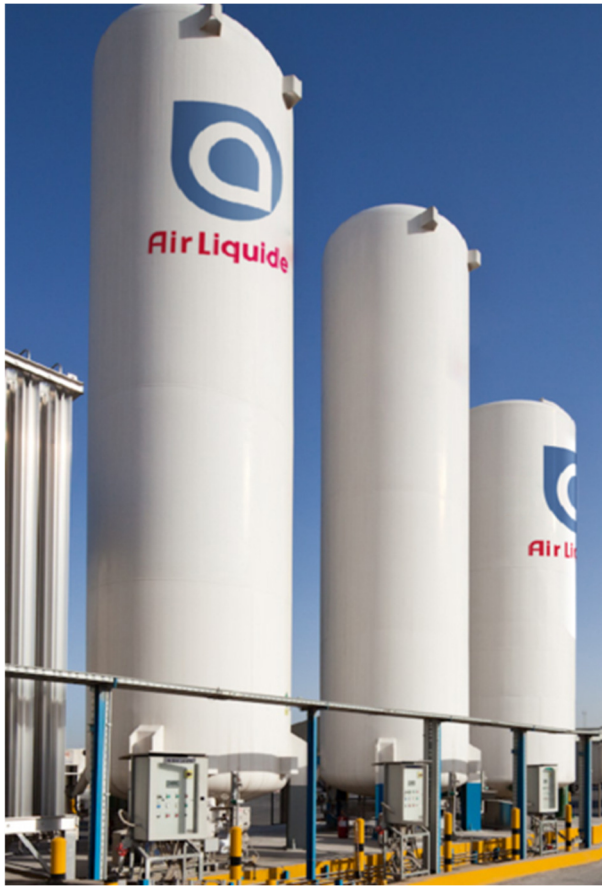
Figure 3-8: Cryogenic storage tanks – vertical tanks.
