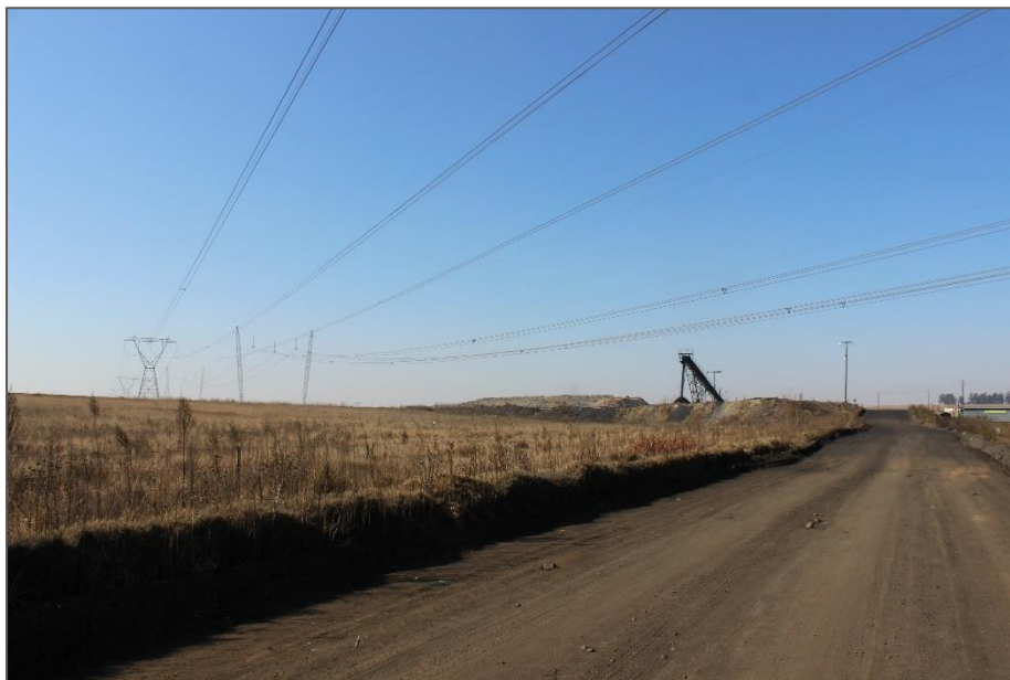
Figure 19: High voltage power lines in the southern sector of the combined study area (Mine infrastructure and dump in background).
