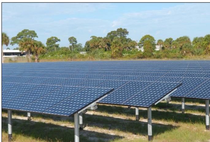
Figure 1.3. Stationary solar PV panels.
