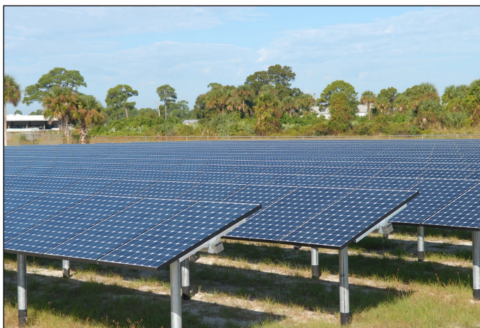
Figure 1.3. Stationary solar PV panels.
