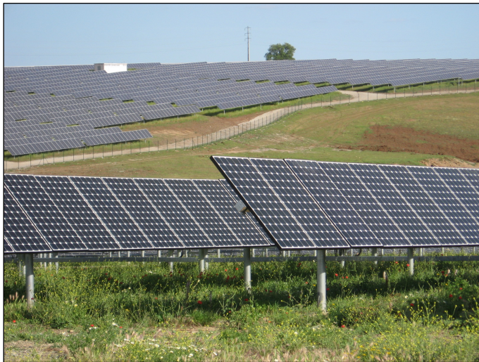
Figure 1.2. Photovoltaic (PV) energy facility.
