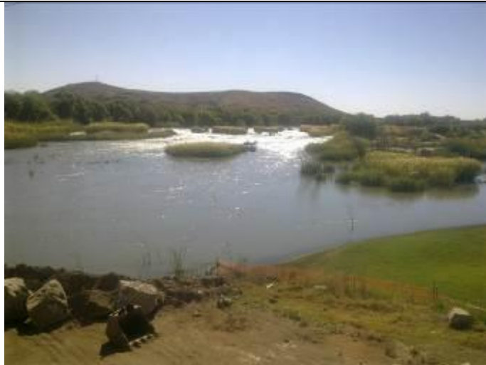
Figure 14: Upstream view of the C3 site, indicating some construction activities at the site.
