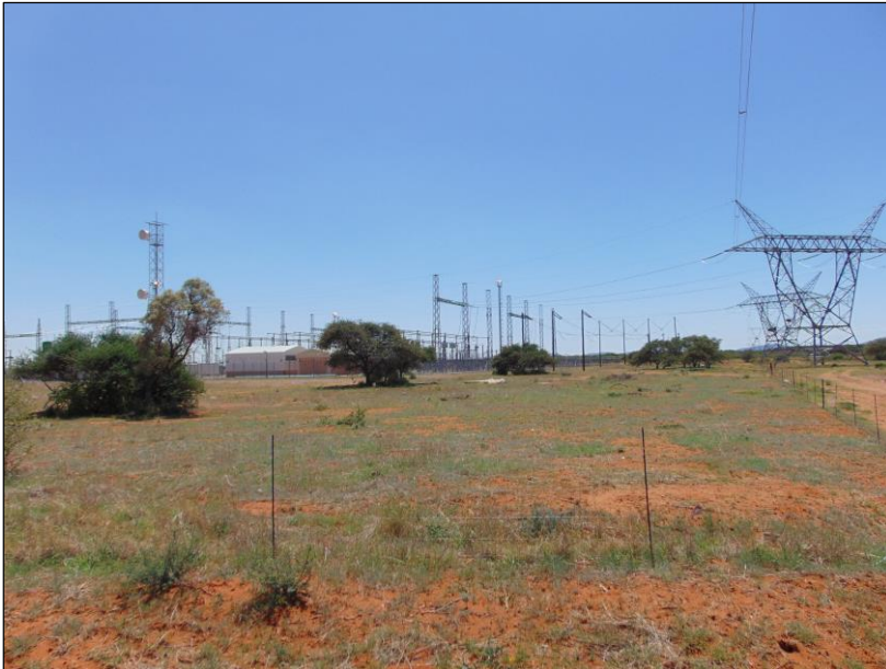
Photograph 1.4.3. Overview of the Eskom substation from the road.
