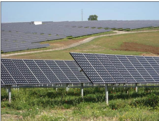
Figure 1.2. Photovoltaic (PV) energy facility.
