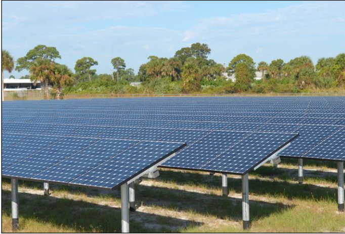
Figure 1.3. Stationary solar PV panels.
