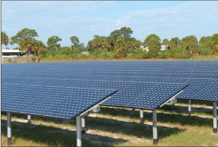
Figure 1.3. Stationary solar PV panels.
