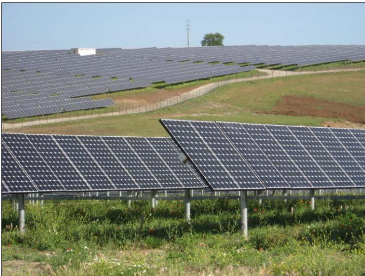
Figure 1.2. Photovoltaic (PV) energy facility.
