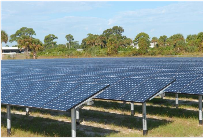
Figure 1.3. Stationary solar PV panels.
