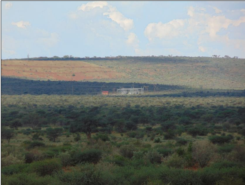
Photograph 1.4.3. Overview of the Eskom substation situated East of the Tshepo SPP site.
