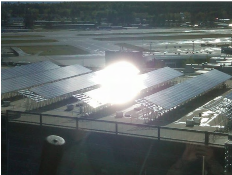
Plate 6, Glare experienced in the Control Tower at Boston Regional Airport from a PV array
