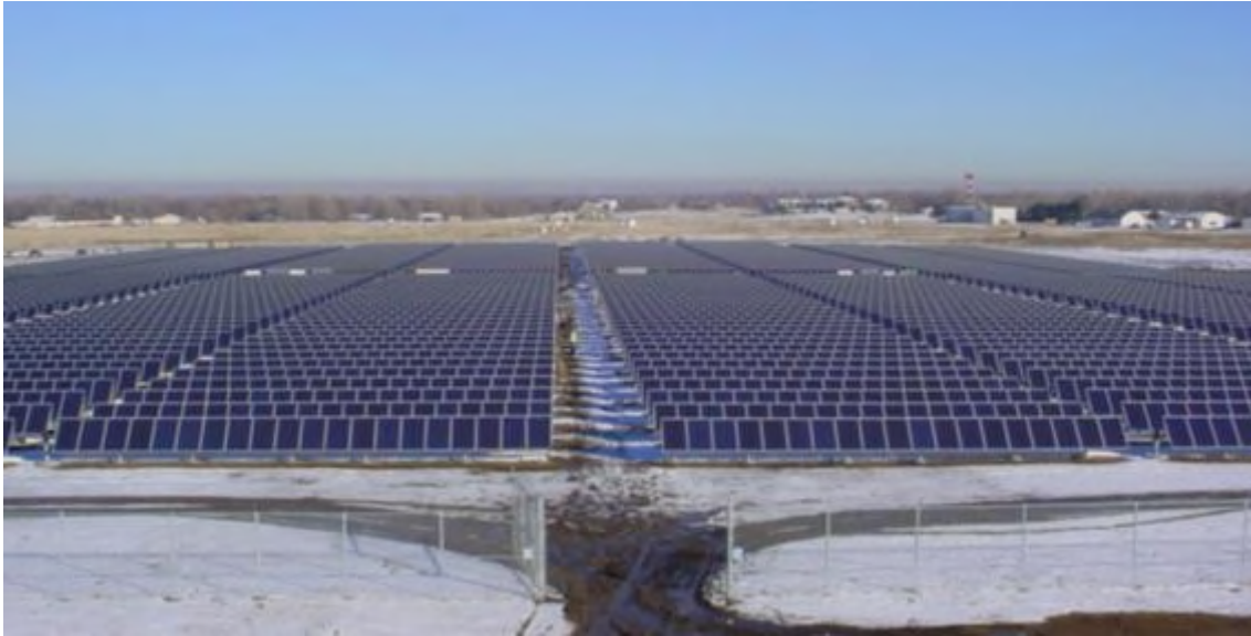
Plate 3, PV array viewed from above. Note the array rows are read as one and have a similar impact as the roof of a large industrial building might.
