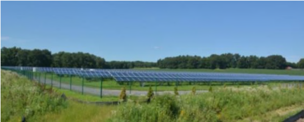
Plate 2, PV array viewed from approximately the same ground level as the array. Note the array appears as a linear dark element in the landscape
